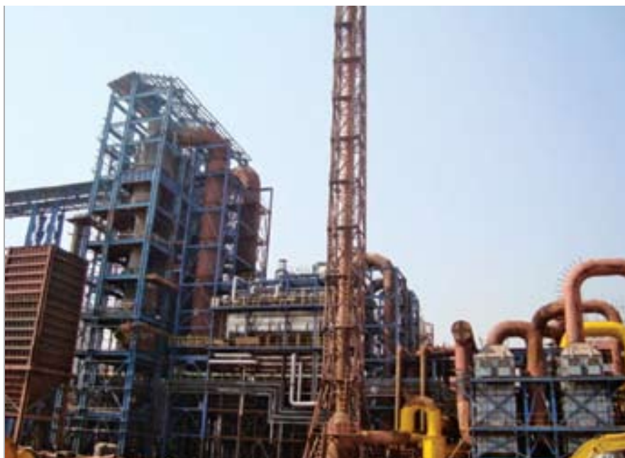
Coal to Gas plant at Iron Ore Pelletisation plant, Barbil
