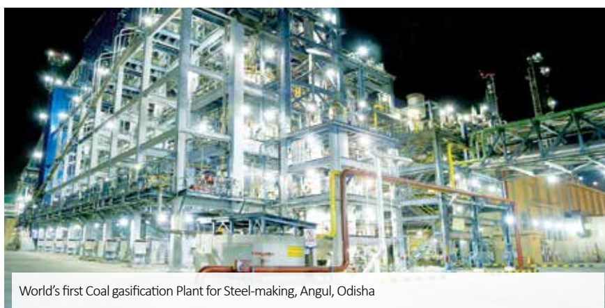
135X6 (810) MW Captive Power Plant, Angul, Odisha
